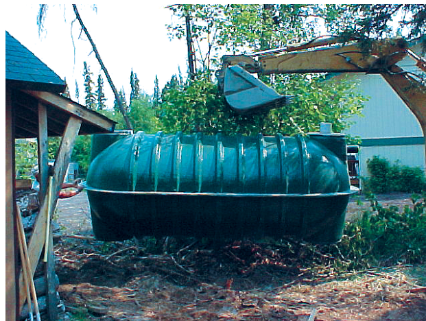
Orengo Fiberglass Tank being installed as part of an AdvanTex Treatment System
