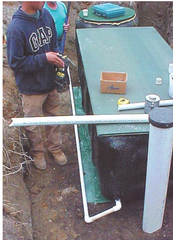
Transport Line flows from the Riser to the Filter. This line slopes to drain back to the tank.
