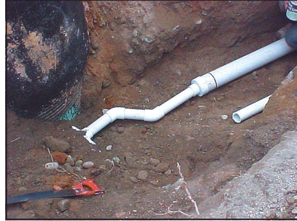
Discharge Line flows from the Riser to the drain-
